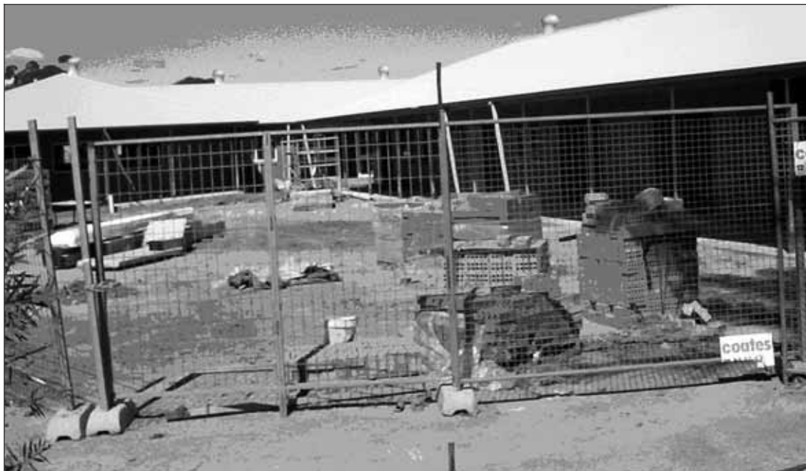
ALMOST DONE: The new buildings under construction at St Patrick's PS, Cessnock.
