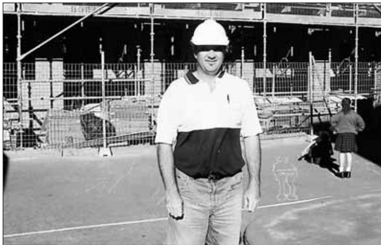
WORK IN PROGRESS: Greg Procter, construction supervisor, stands in front of the new building at St John's PS, Lambton.
